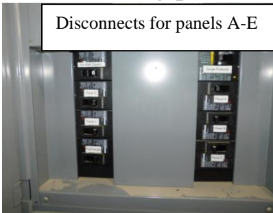
Panel A W/39 breakers
