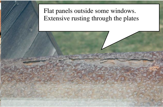
Extensive rusting to flat panels on the roof top
